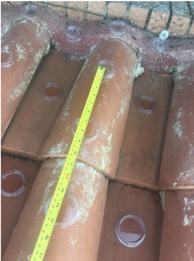
Figure 14. Empty dishes fixed on the North roof.
