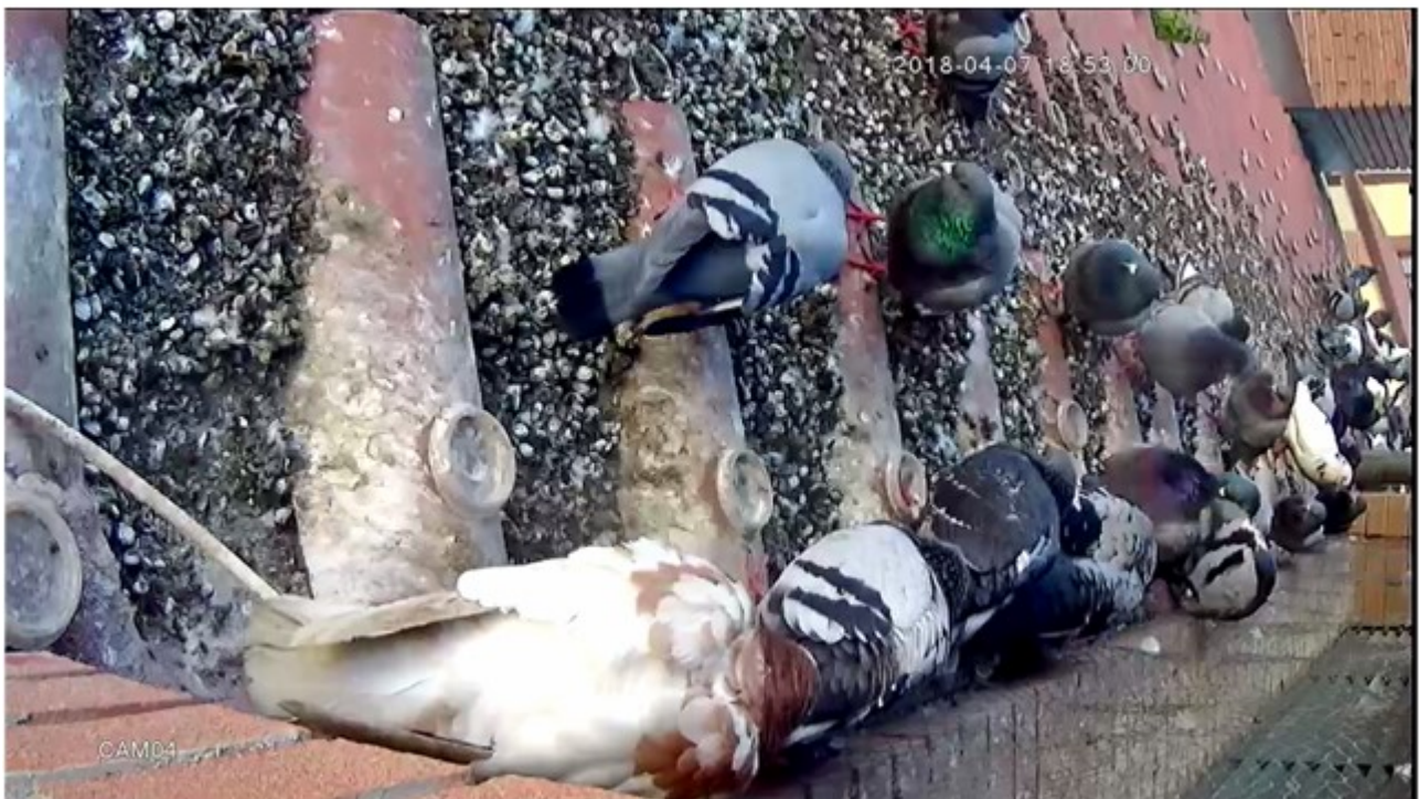
Figure 19. North Roof provided with Empty Dishes. The picture has been taken at the sunset after about 1 year from the installation.
