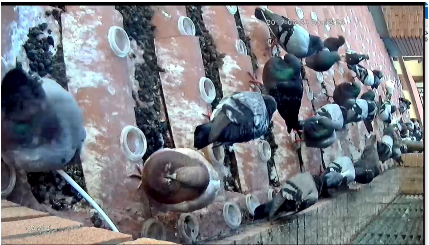
Figure 17 North Roof provided with Empty Dishes. The picture has been taken at the sunset (Day 90).
